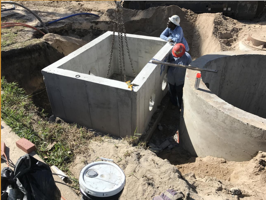
Valve Vault Setting
