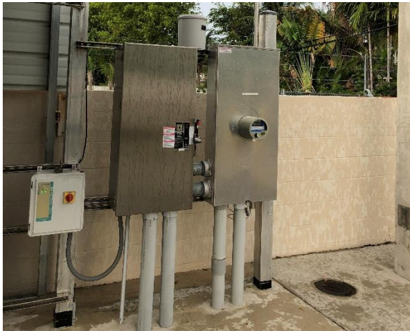
Electric Control Panel
