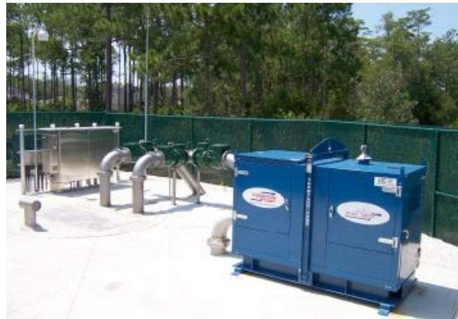
Bypass Pumping Unit
