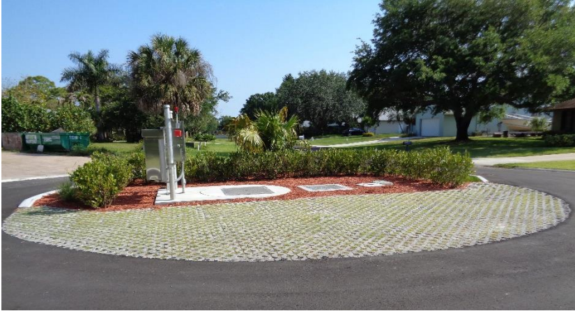
Lift Station Example
