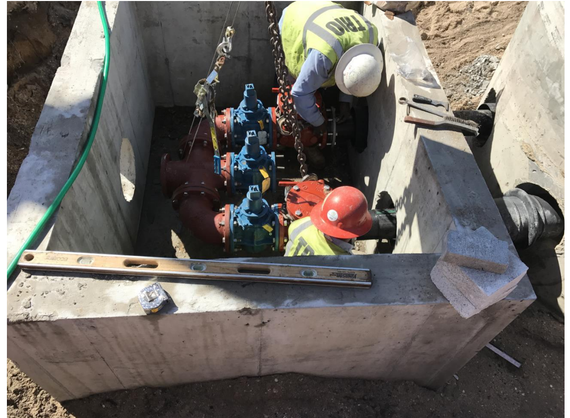
Piping within Valve Vault
